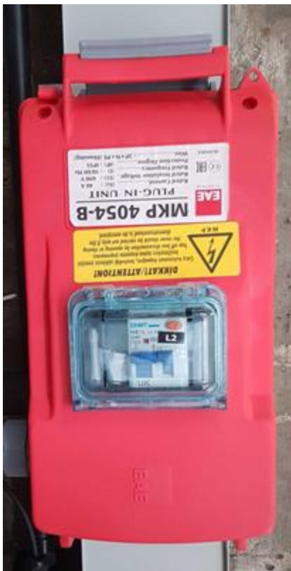
Figure 27. Tap-off Box fitted to Busbar (Front)
