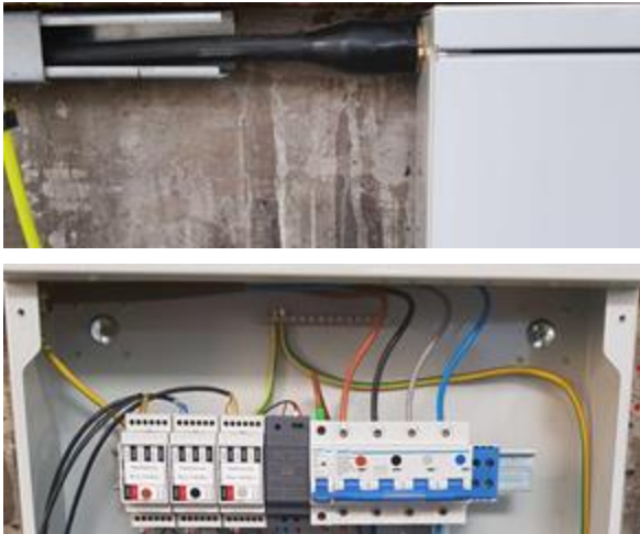
Figure 4. Supply to Distribution Board
