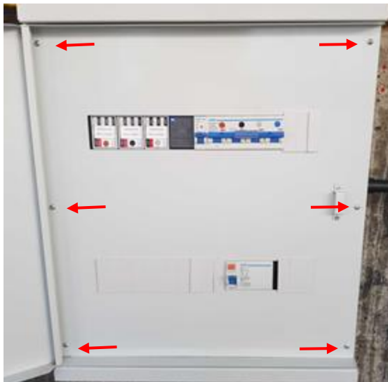
Figure 1. Array Circuit Distribution Board
