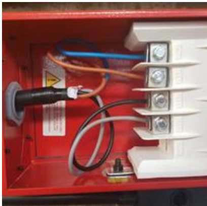
Figure 5. Wiring of Busbar Feeder Unit
