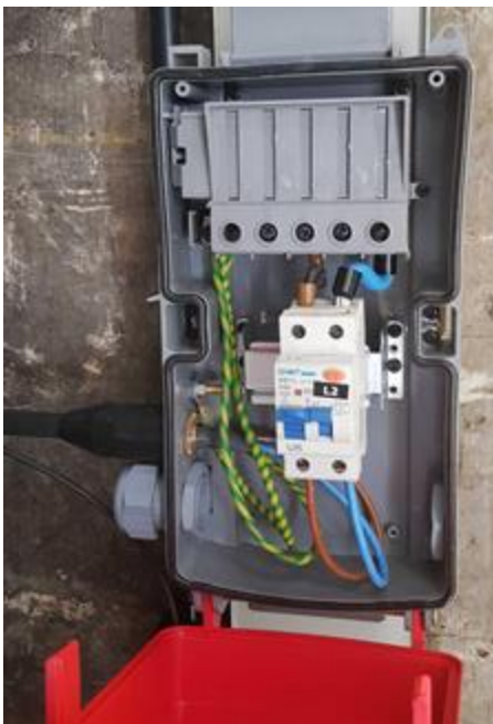
Figure 29. Tap-off Box with L2 connected to RCBO
