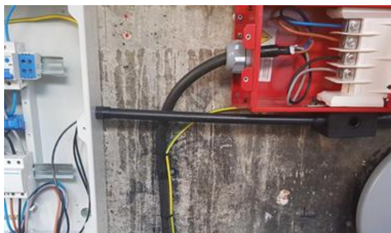
Figure 12. Example Data Cable connection from Distribution Board to first Data Box
