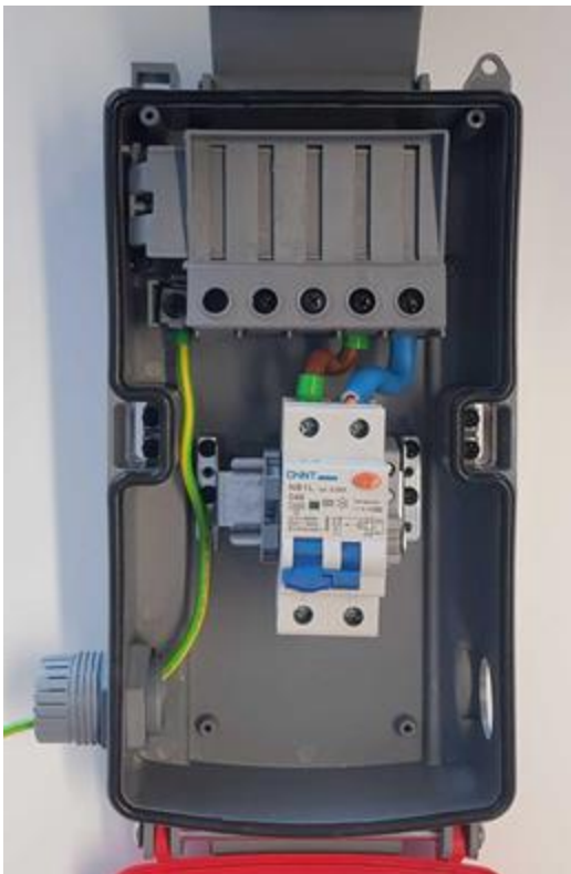
Figure 24. Tap-off Box with L1 connected to RCBO
