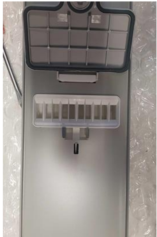
Figure 25. Exposed Tap-off Point, cover to be removed
