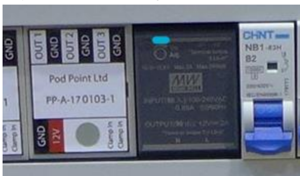
Array controller PSU indicator lamp (normal).
