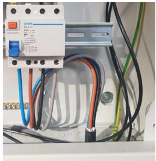
Figure 7. Lower DIN Rail RCCB connected to Busbar Supply Cable
