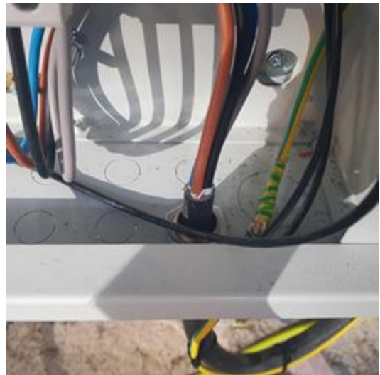
Figure 6. Supply to Busbar gland connection to Distribution Board
