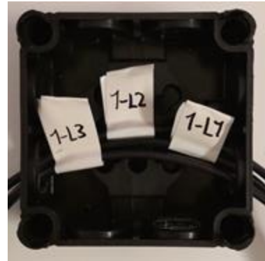
Figure 21. First set of Data cables in Data Box
