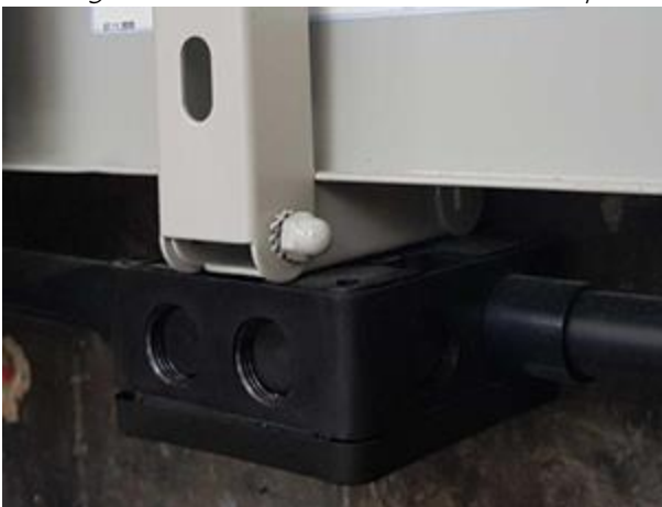
Figure 20. Example Conduit fitted to Data Box
