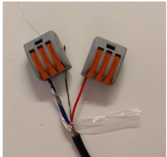
Figure 30. Incoming Data cables as if fitted to a unit, only showing 1 phase pair of Data Cables for clarity
